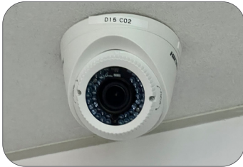
Figure 1: Dome camera mounted on an indoor ceiling
