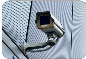
Figure 2: Bullet camera mounted on an exterior wall
